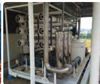
Crown Embalagens / SP Osmose Reversa 40 m 3 /h
